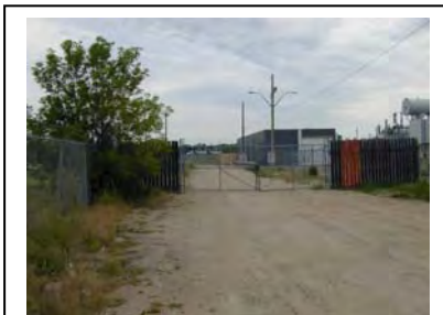
Electric Substation in Riversdale
